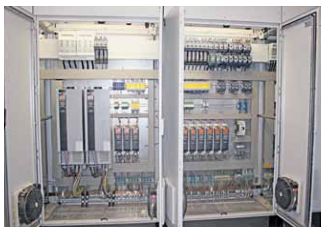
»6a/b Control engineering for preparation in a backing brick plant
